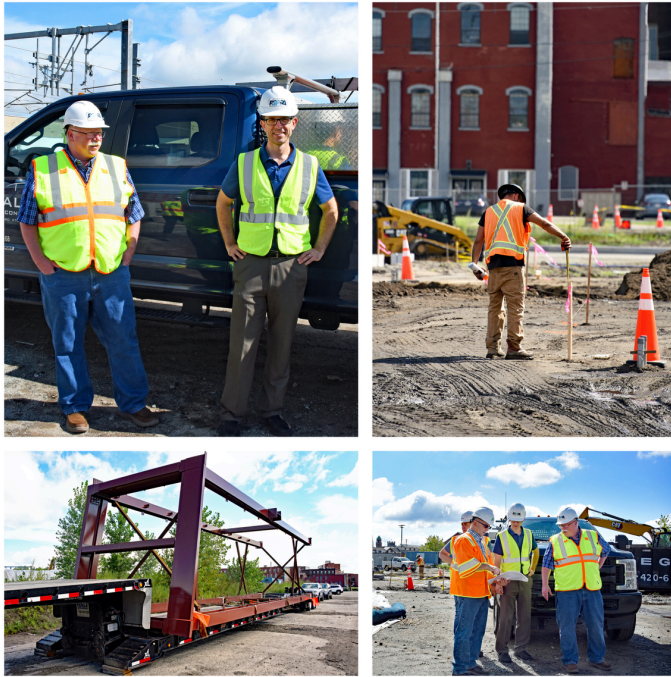
Clockwise from upper left: RIPTA Project Manager James Canty and RIPTA Principal Planner Greg Harris on site at the transit center construction site, staking out boundaries, RIPTA team looking over plans with RIDOT managers, framework for elevator shaft.
